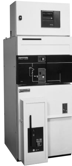
Fig. 4: EMC application example: a medium-voltage SM6 panel containing a circuit breaker designed to interrupt power (hundreds of amperes under tens of kilovolts), and a SEPAM programmable control, monitoring and protection unit. The complete assembly must remain operational under all circumstances.
